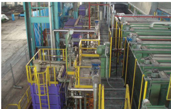
Fig 2 Air jet headers with water headers in between during installation in the cooling section of the furnace
